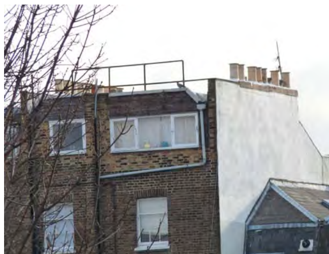
Ugly roof extension
