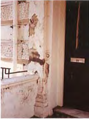
Example of badly deteriorating mid 19 th C stucco in the Westbourne area (photo 1988)
