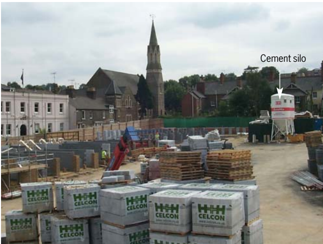
Figure 4 View of a construction site showing plastic-wrapped palletised materials in the foreground and a cement silo towards the rear of the site
