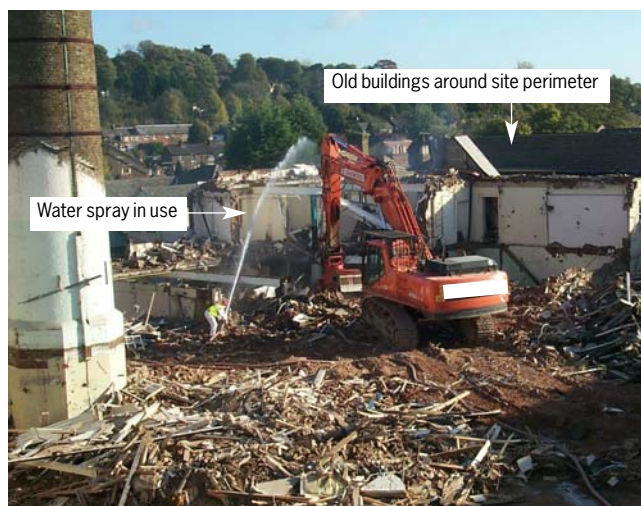
Figure 2 Old buildings around the site perimeter waiting to be demolished can provide effective screening against pollution crossing the site boundary
