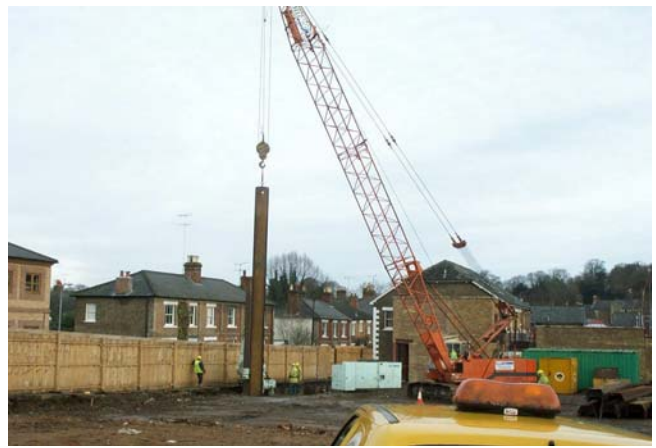
Figure 9 Crane lifting pile into position for driving (piling can cause high levels of noise and vibration to be generated)
