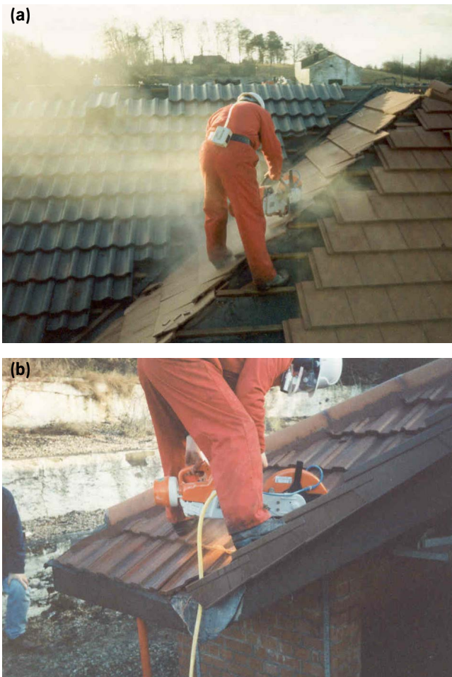
Figure 2 (a) A circular saw generating dust when cutting roof tiles, (b) the same circular saw using a water spray when cutting tiles. Courtesy of Marley Building Materials
