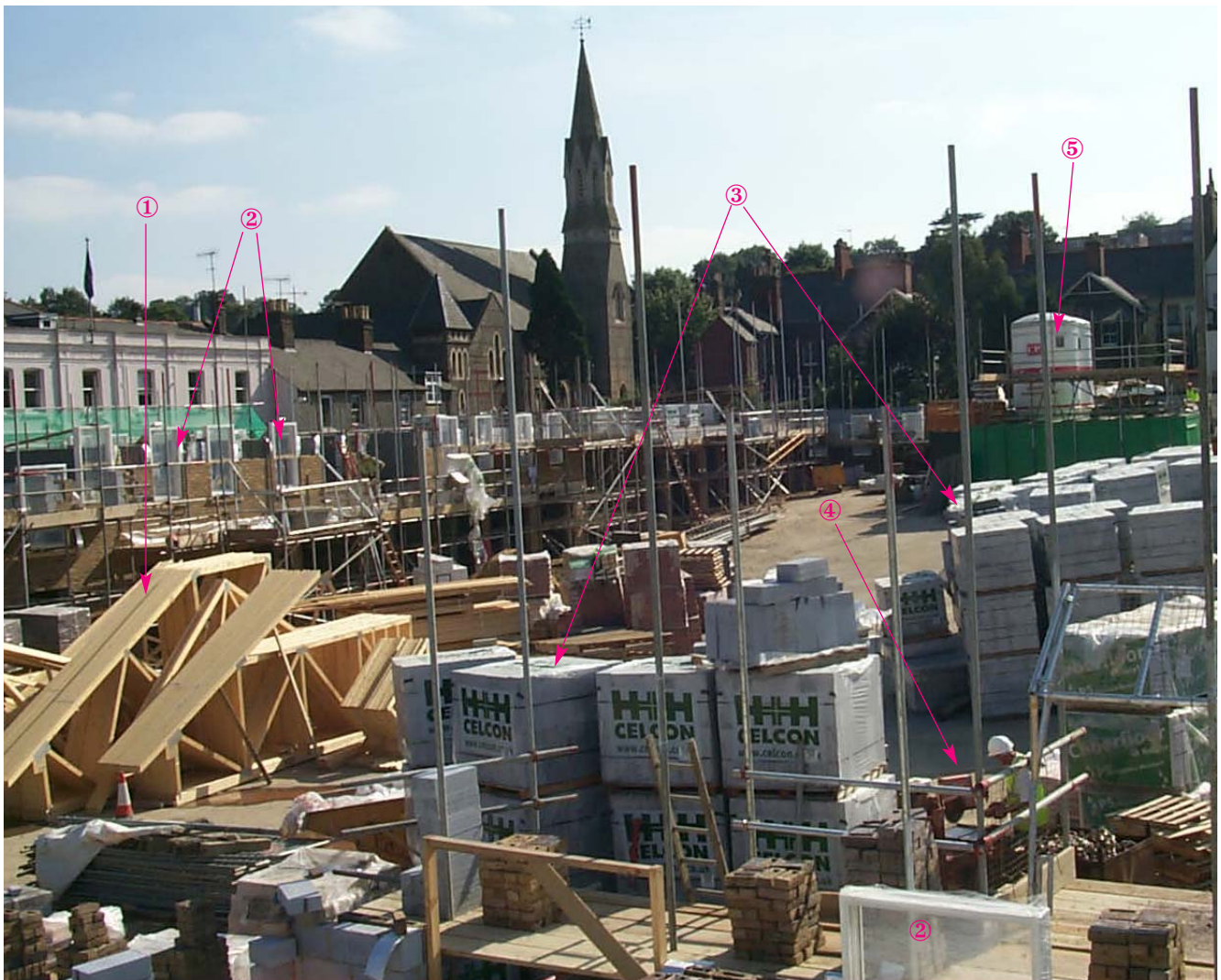
Figure 3 Examples of good practice: ① = prefabricated roof timber sections; ② = prefabricated window frames; ③ = bricks and blocks polyethylene-wrapped until required; ④ = bench-mounted cutter with water dust suppression; ⑤ = cement silo
