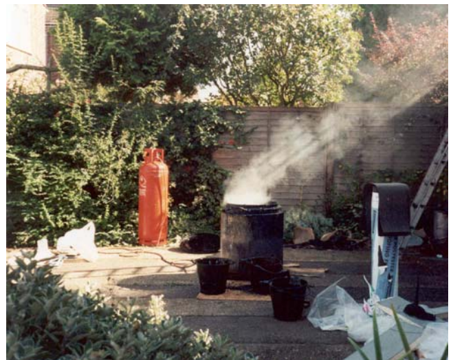
Figure 4 Uncovered tar boiler emitting vapour. Courtesy of Envirobods Ltd
