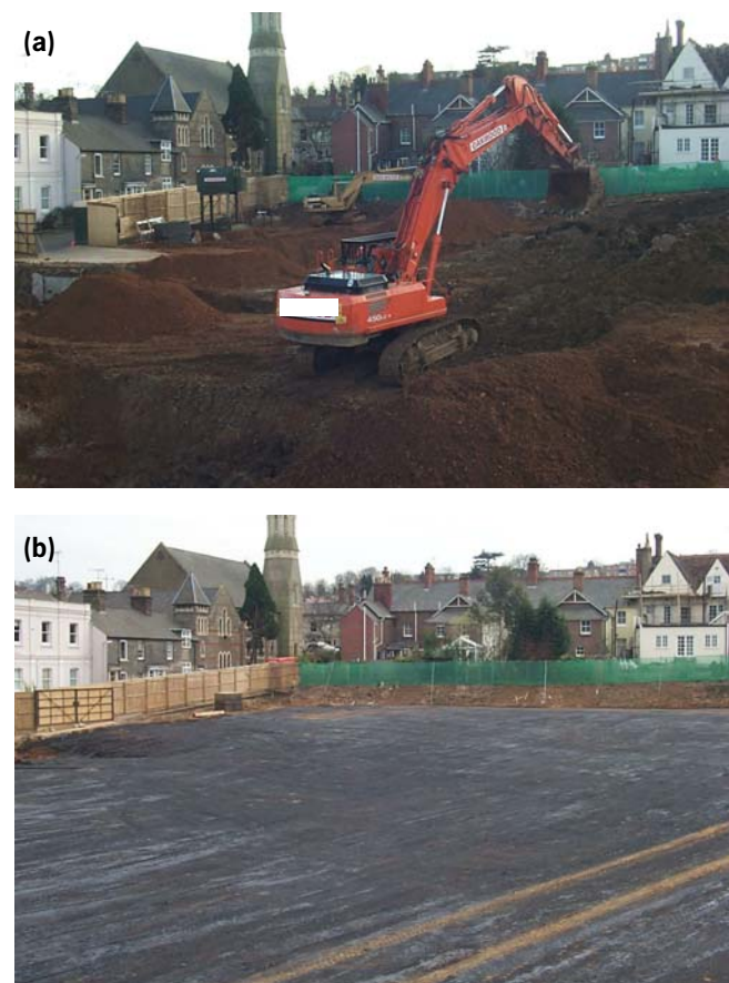
Figure 8 (a) Earthworking activities at a typical construction site, (b) same site after levelling and stabilising, and before foundation and service laying
