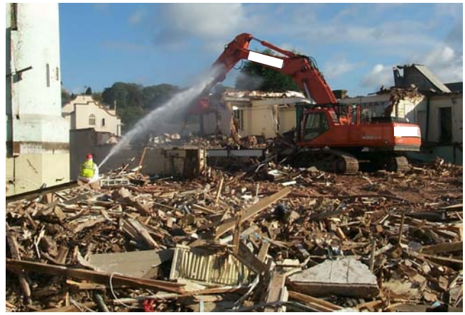
Damping down demolition activities with water sprays minimises dust emission and spread
