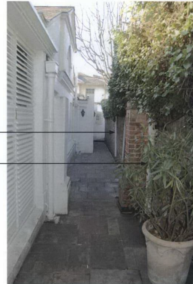
Photo of leaning garden wall
