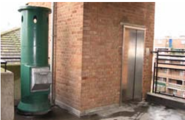
Refuse chute at top floor level
