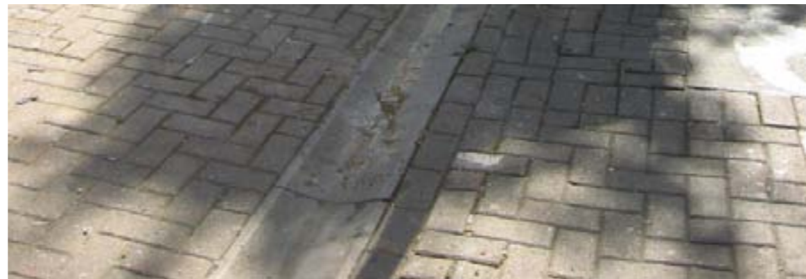
Dull block paving
