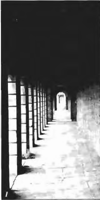
1 As open, 'unoccupied' structures, the Great Circle and arcades are particularly susceptible to weathering
