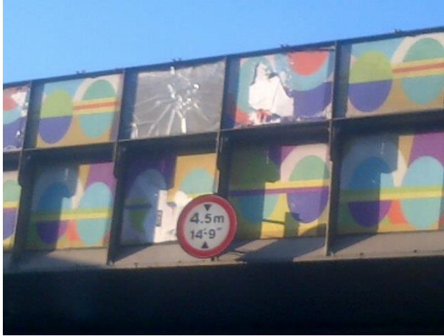
The damaged panels
