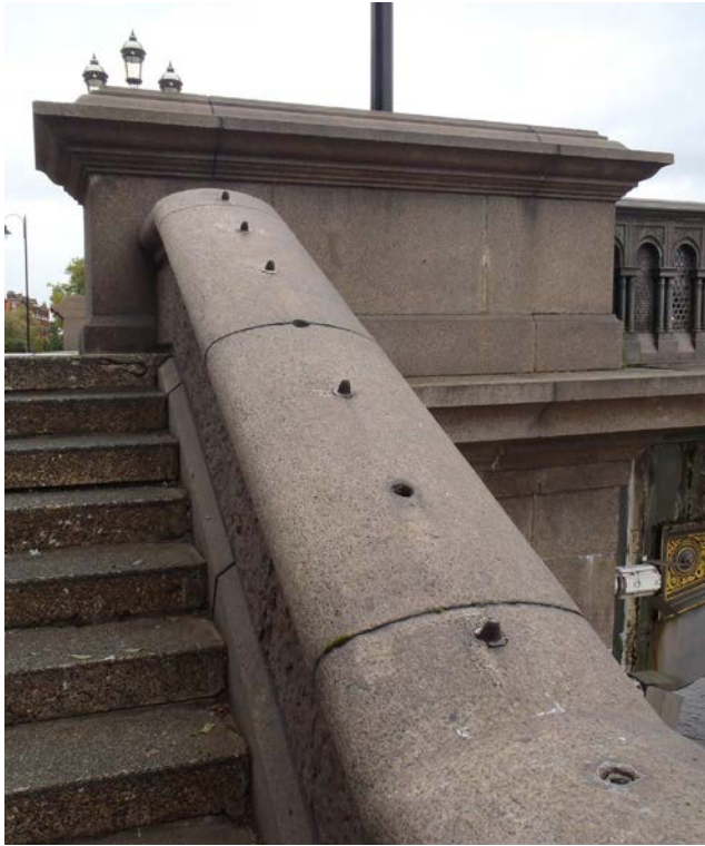
Missing metal studs on top of retaining wall
