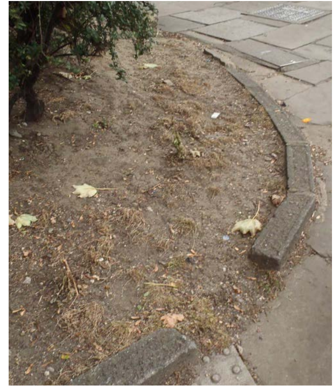
Poorly matched concrete coping stones
