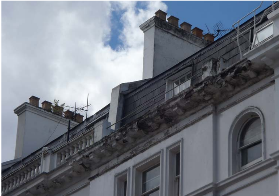
Lack of repairs and maintenance to bracketed cornice
