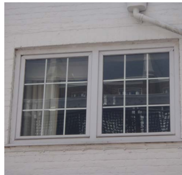
Inappropriate uPVC windows
