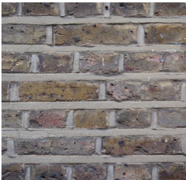
Inappropriate weather struck pointing
