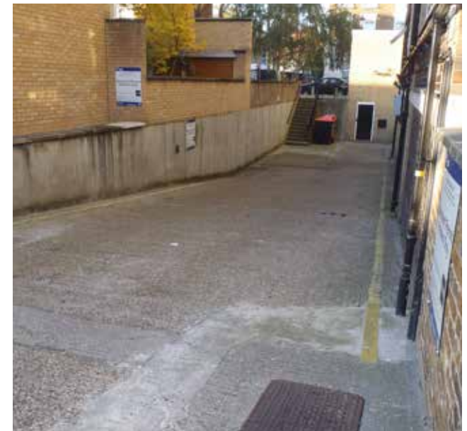
Ramp at Crossways House ignoring the historic building line
