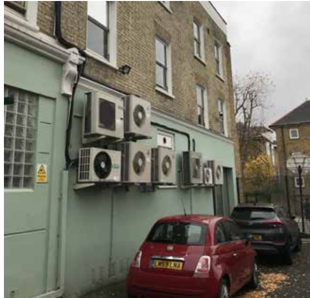
Air conditioning units not hidden from view
