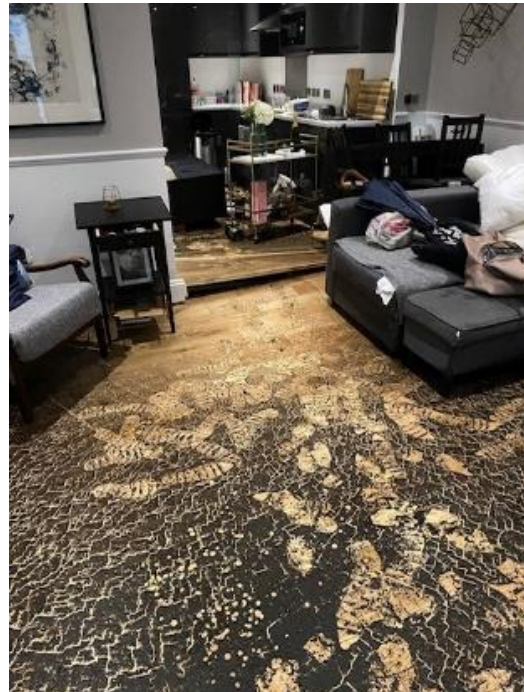
Figure 9-8: Damages to properties due to flooding (images reproduced from residents' responses to the RBKC questionnaire). Top left: Colville Road; Top right: Norland Square; Bottom left: Holland Park Avenue; Bottom right: Warwick Road.
