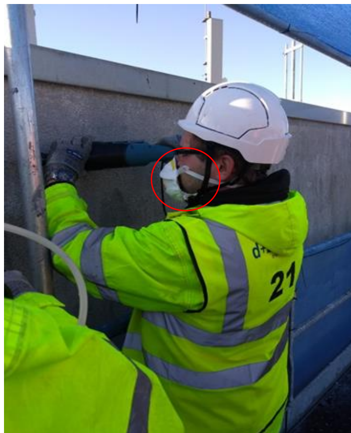
Image showing the poor fitting of the RPE indicated by the visible gap
